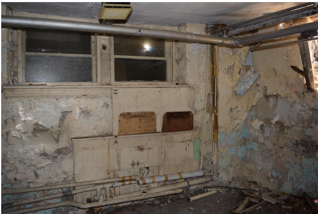
Figure 46: View facing north of the 'Boys' bathroom showing the former location of sinks (May 2016).
