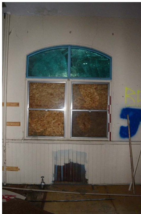
Figure 57: Former hot-water radiator location, wainscoting, chair rail, and window trim in the east first-level classroom (May 2016).
