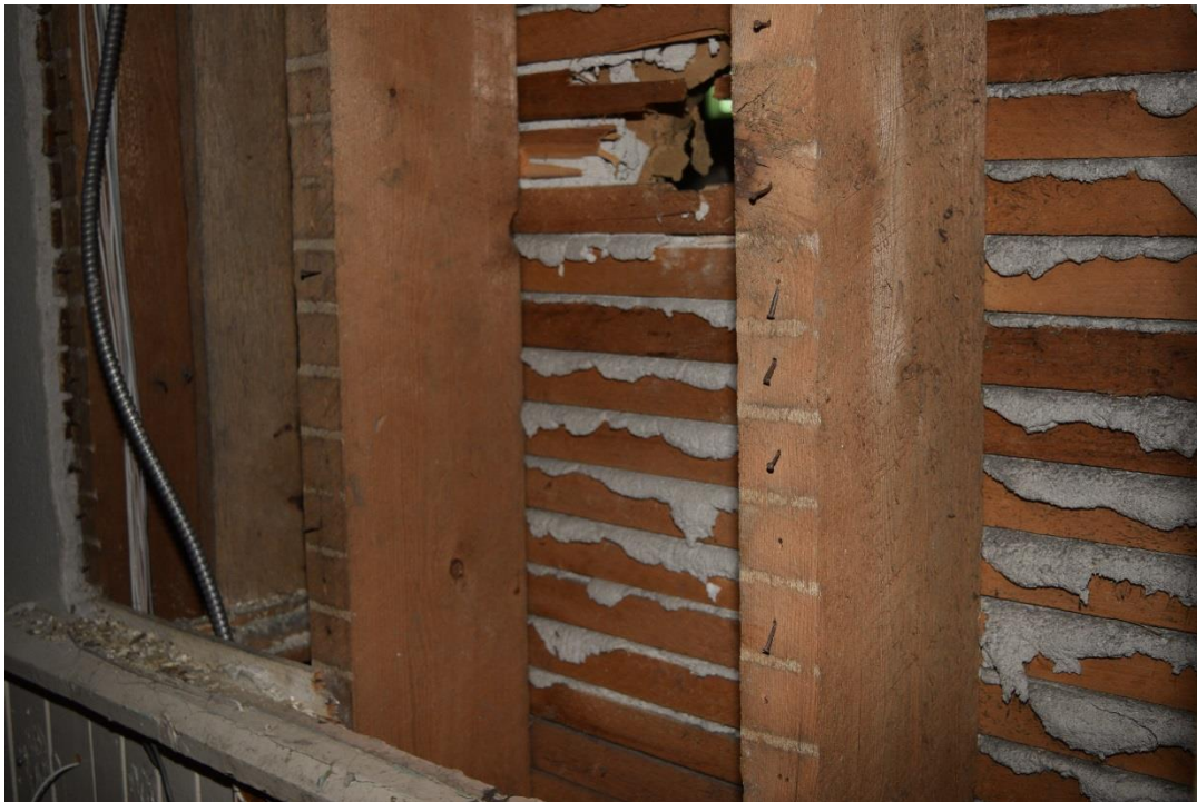
Figure 67: Plaster 'keys' as seen in the second-level classroom (May 2016).
