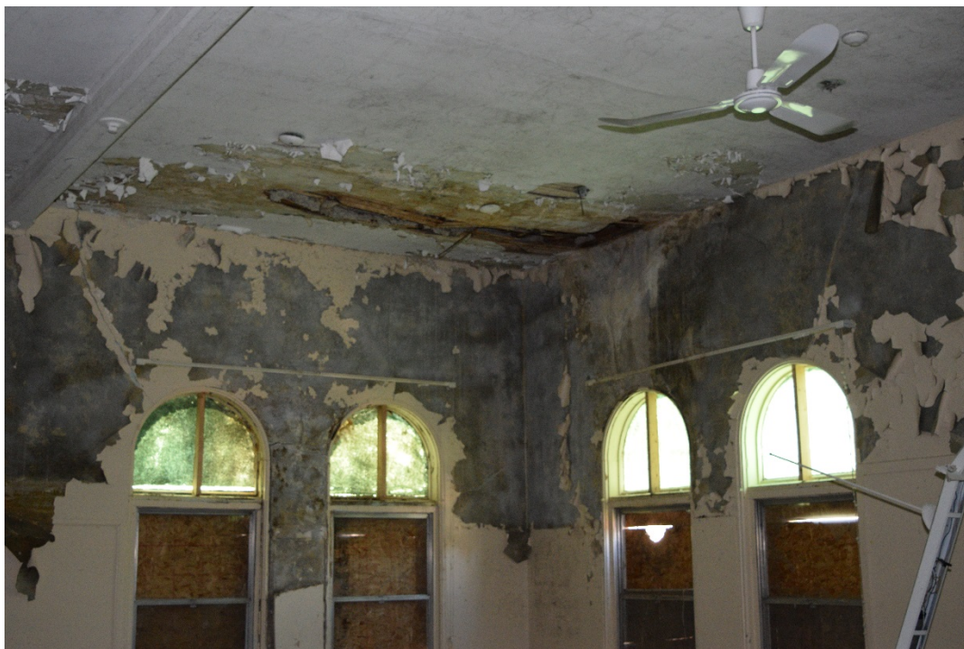
Figure 70: Water damage in the northwest corner of the west second-level classroom (May 2016).
