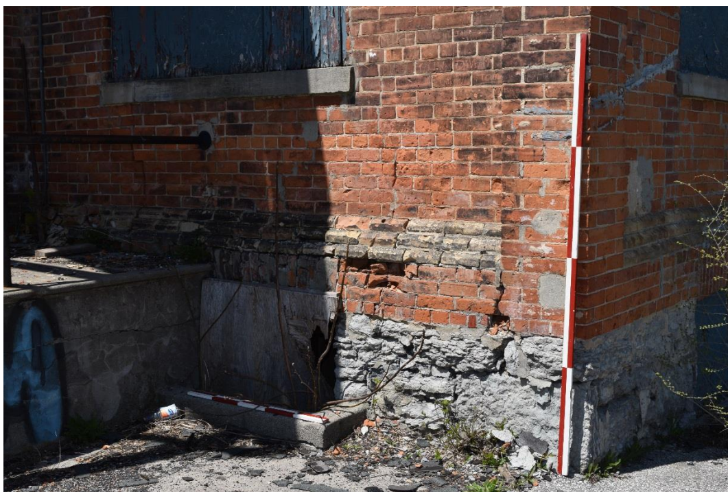
Figure 72: Erosion, exfoliation and spalling of the brick and stone construction on the southeast corner of the main block (May 2016).
