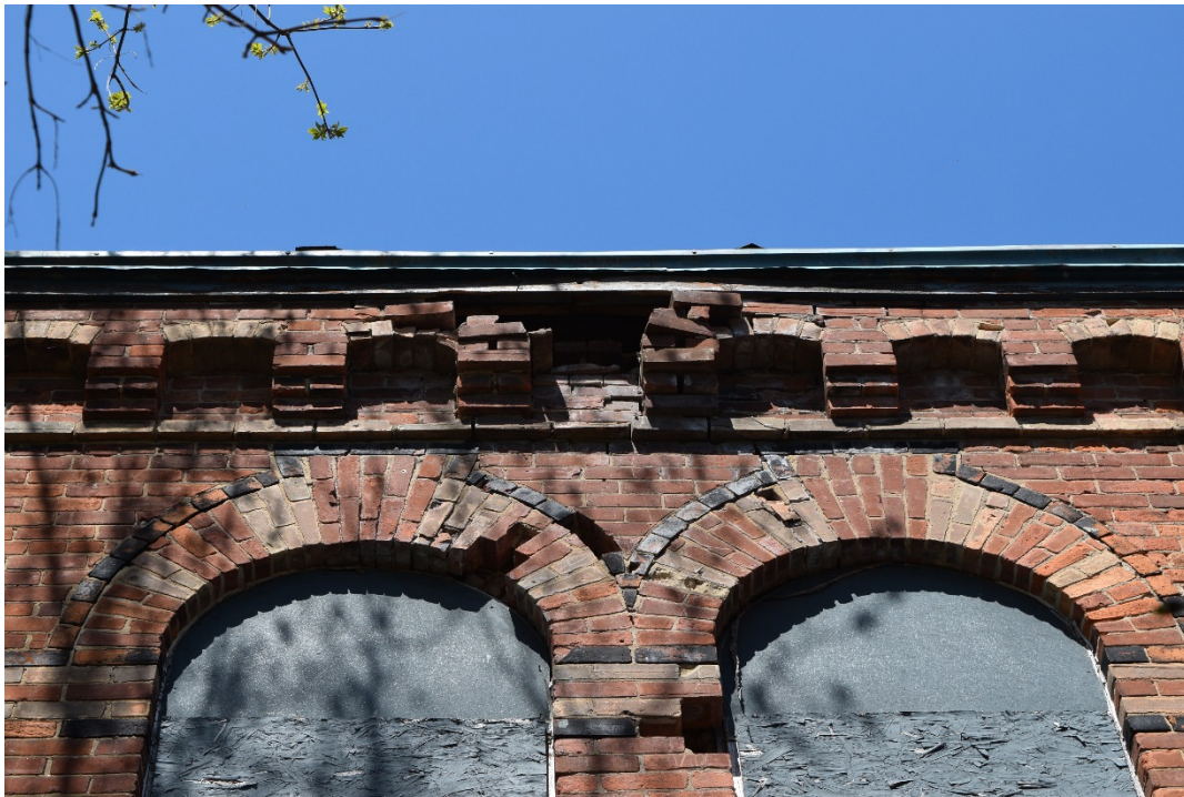
Figure 72: Missing and displaced section of arched corbel table, voussoir, and window column on the southwest façade of the main block (May 2016).
