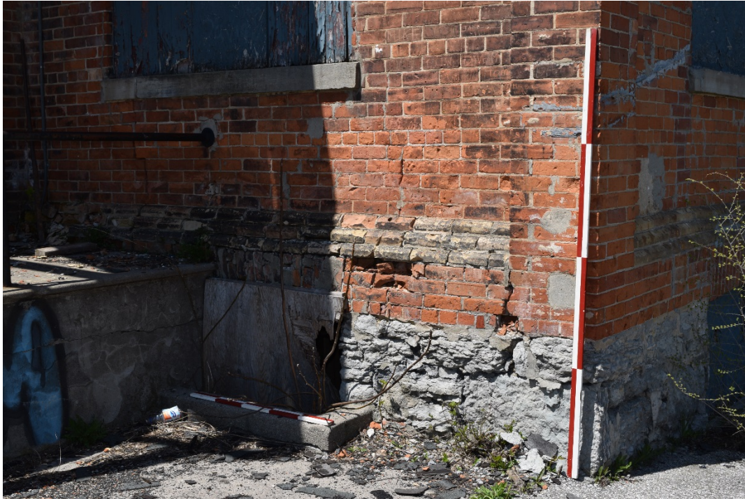
Figure 73: Erosion, exfoliation and spalling of the brick and stone construction on the southeast corner of the main block (May 2016).
