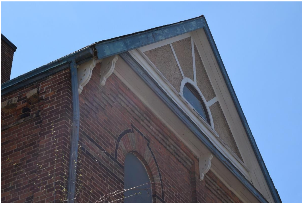
Figure 37: Grooved and perforated quarter-round brackets at the eaves and pent roof of the north transept (May 2016).
