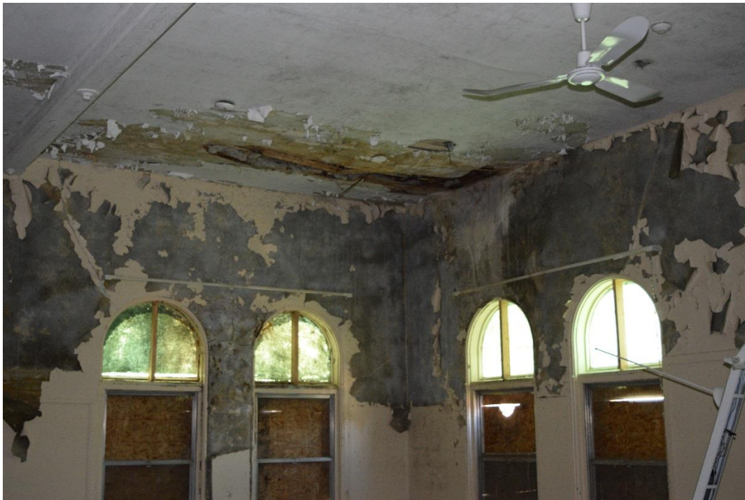
Figure 69: Water damage in the northwest corner of the west second-level classroom (May 2016).
