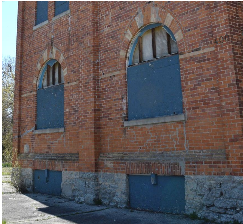
Figure 34: Diocletian windows on the east end wall of the main block (May 2016).
