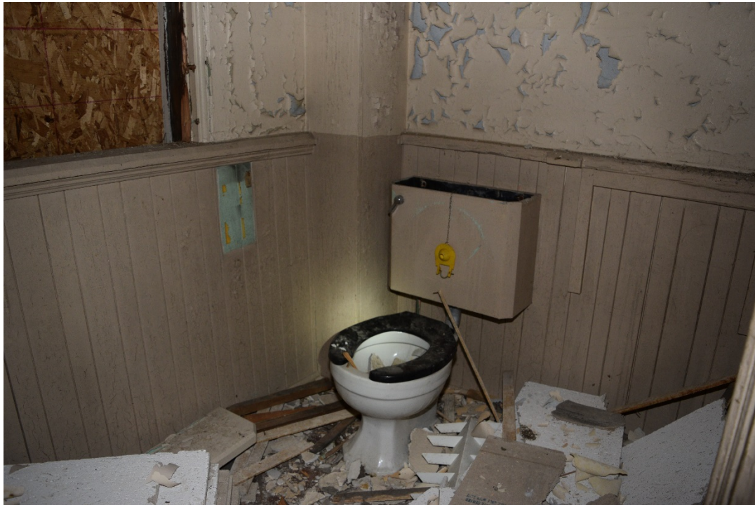
Figure 52: Toilet in the first level of the north transept, facing northwest (May 2016).
