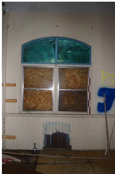
Figure 56: Former hot-water radiator location, wainscoting, chair rail, and window trim in the east first-level classroom (May 2016).
