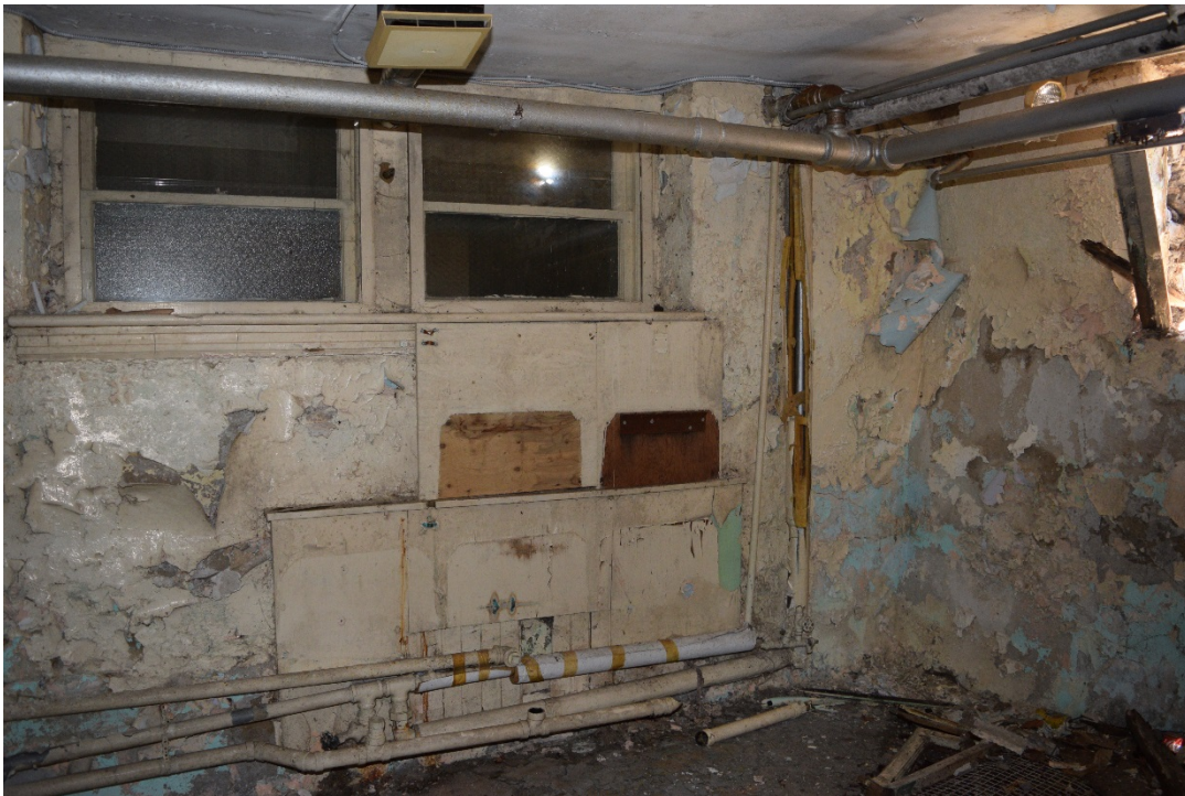
Figure 47: View facing north of the 'Boys' bathroom showing the former location of sinks (May 2016).
