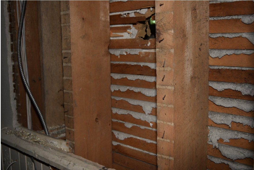
Figure 68: Plaster 'keys' as seen in the second-level classroom (May 2016).
