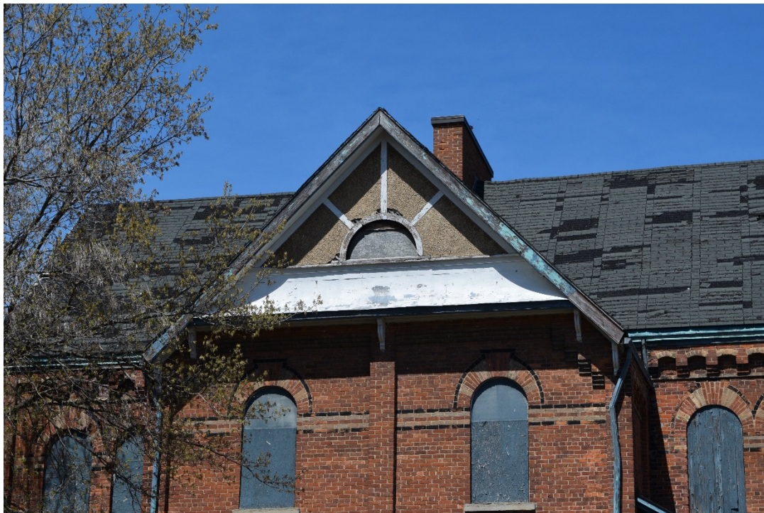
Figure 40: 'Sunburst' Stick decoration and pent roof on the south transept cross-gable (May 2016).
