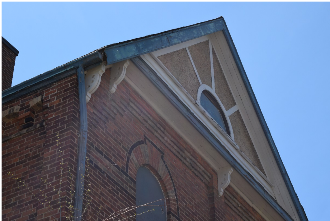
Figure 38: Grooved and perforated quarter-round brackets at the eaves and pent roof of the north transept (May 2016).
