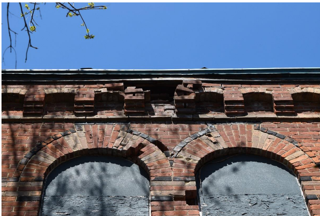
Figure 71: Missing and displaced section of arched corbel table, voussoir, and window column on the southwest façade of the main block (May 2016).
