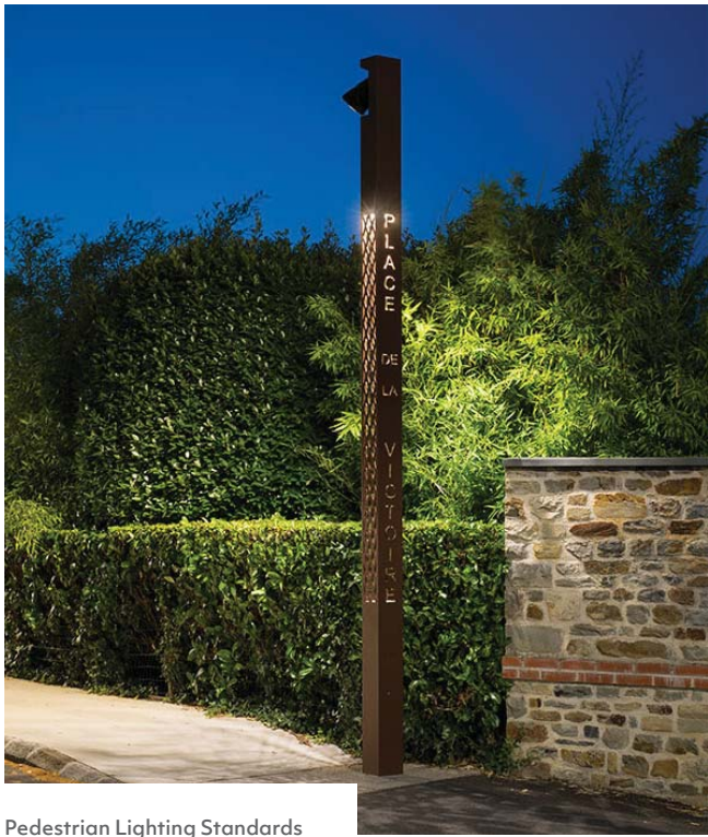
Pedestrian Lighting Standards
