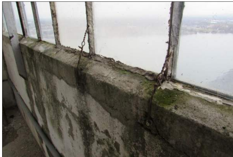
Figure 20: Multiple Repairs at Window Sill in Shipping Tower
