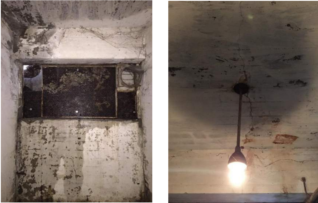
Figure 7 a, b: Perimeter wall and ceiling concrete leak and deterioration
