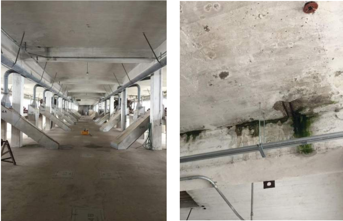
Figure 11 a, b Bin floor structure and localized roof leakage
