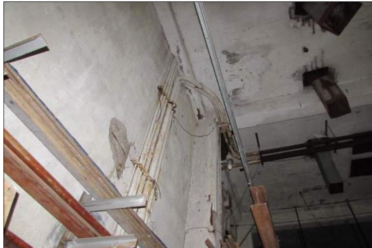
Figure 13: Spalling of Reinforced Concrete Wall Adjacent Storage Bins
