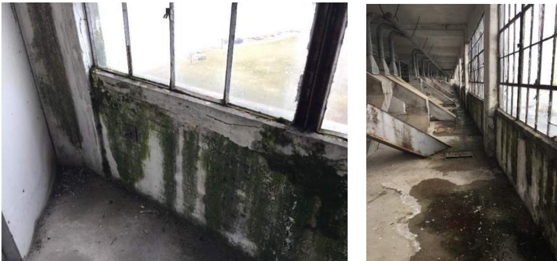
Figure 12 a, b: Bin floor perimeter wall leakage and deterioration
