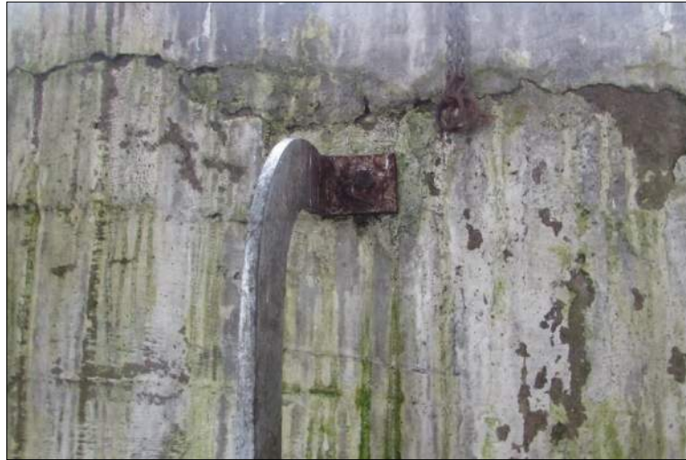
Figure 27: Corrosion of Substation Mezzanine Access Ladder Anchorage
