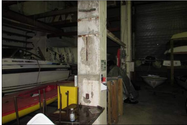
Figure 14: Spalling Observed at Interior Concrete Column in Rail Shed
