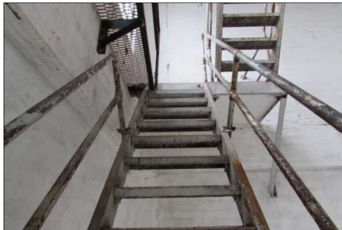
Figure 22: Missing Guard Railing at Floor 3 Mid-Landing of Shipping Tower
