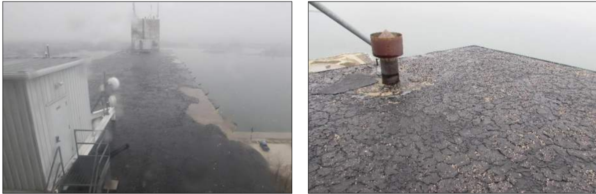
Figure 33a, b: Upper roof membrane failure
