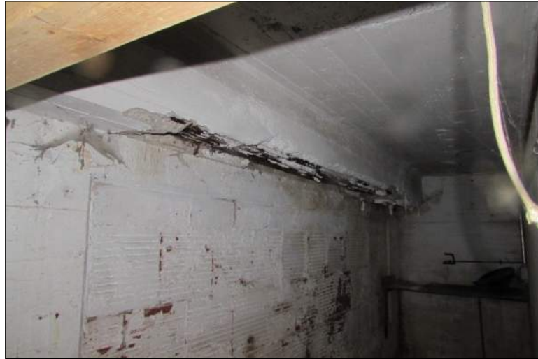
Figure 15: Damaged Reinforced Concrete Beam in Basement (Shop) below Warehouse
