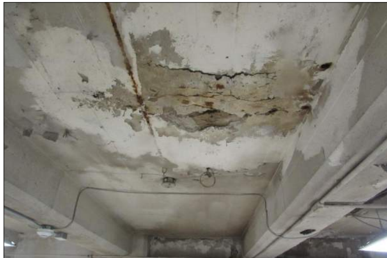
Figure 16: Very Severe Deterioration of the Suspended Slab in Basement (Shop) below Warehouse
