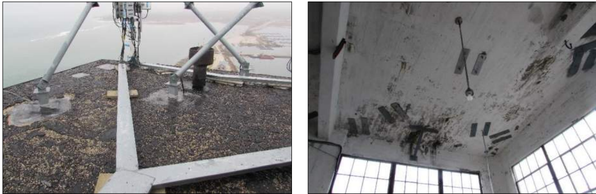
Figure 30a, b: Roof Top Equipment Anchorage in Shipping Tower
