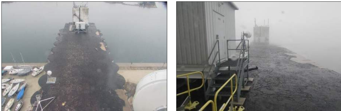
Figure 31a, b: Primary roof without fall arrest system
