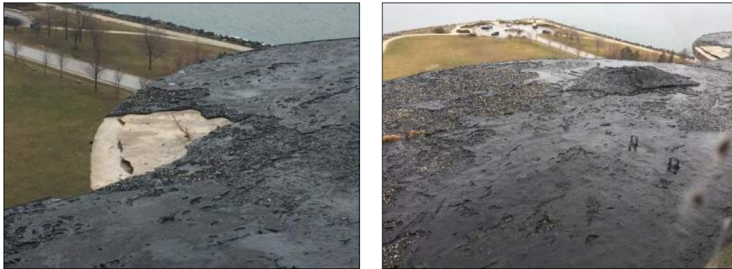
Figure 34a, b: Bin roof membrane failure
