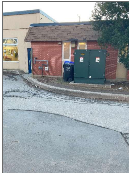
Photograph 1 – Transformer adjacent to northern portion of east wall.
