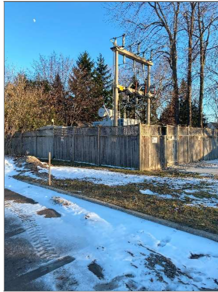
Photograph 9 – Transformer compound to the south, viewed from the northwest.
