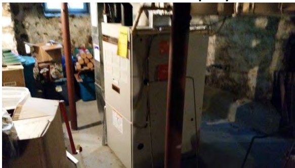
19. View of furnace in basement of the house on 774 Hurontario Street.
