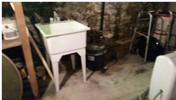
22. View of sump pump in the basement of the house on 774 Hurontario Street.
