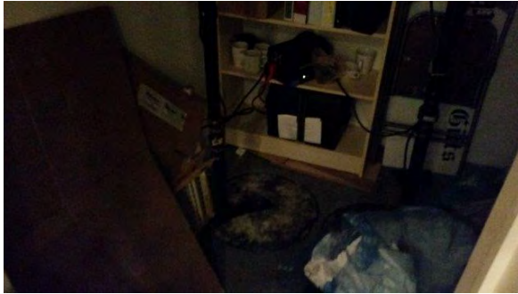
25. View of second sump pump located in the basement of the addition to the house on 774 Hurontario Street.
