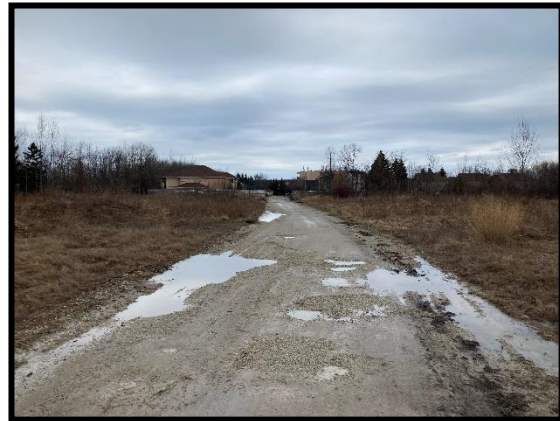
Image 14: Disturbed Area (March 5, 2024; Facing North)
