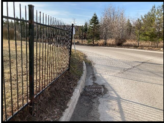
Image 1: Disturbed Area (March 5, 2024; Facing South)
