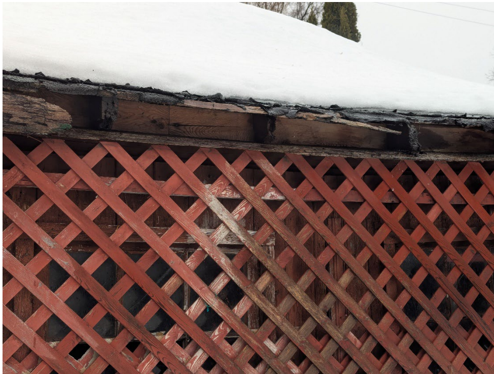
Damaged wood and deteriorated shingles noted at the roofline (west elevation) above.
