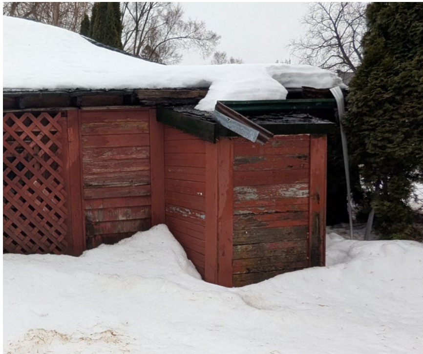
Damaged roof at the small garage rear addition above.
