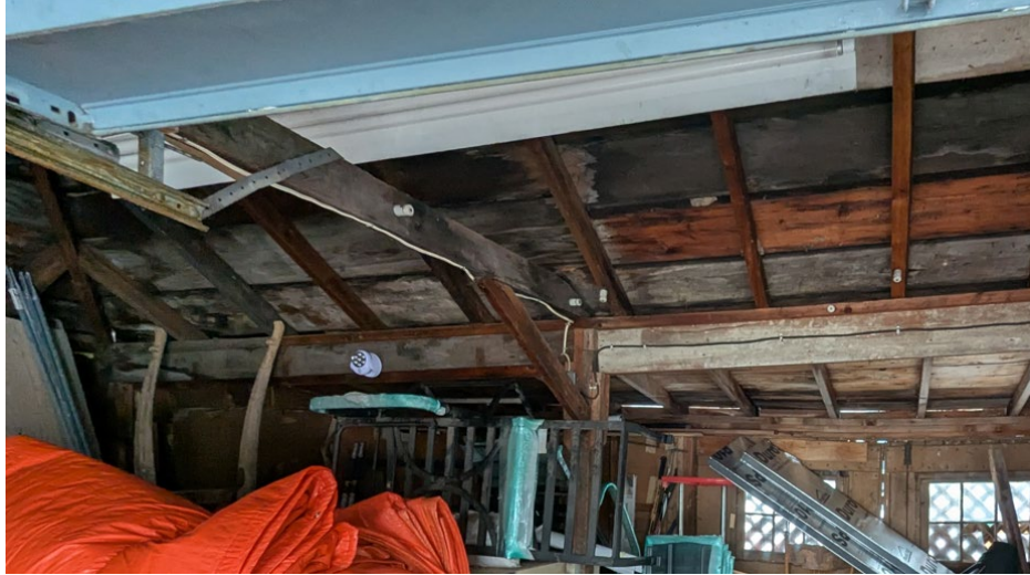
Multiple signs of water damage noted on the interior of the roof above.
